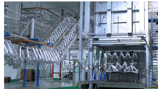
T4 Heat Treatment Furnace
